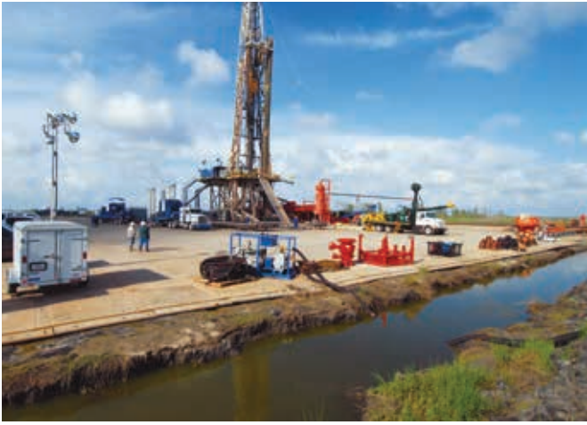
Figure 2. Ground level image of a rig installation on soft soil with DURA-BASE in South Louisiana.
