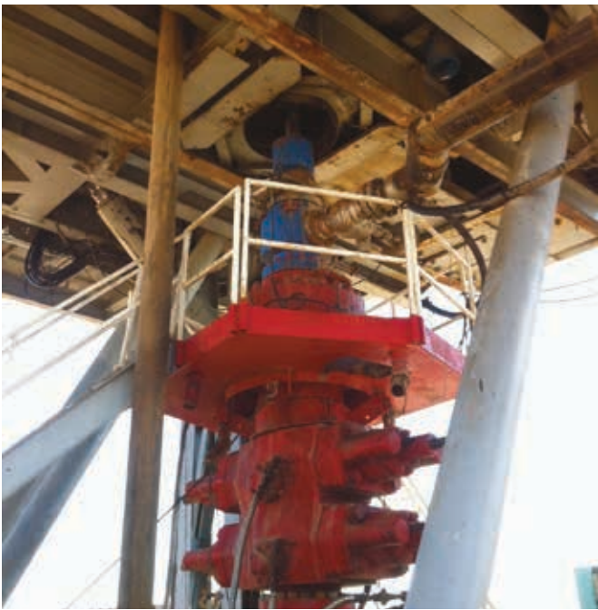
Figure 7. Dual element RCD installed atop a BOP stack.
