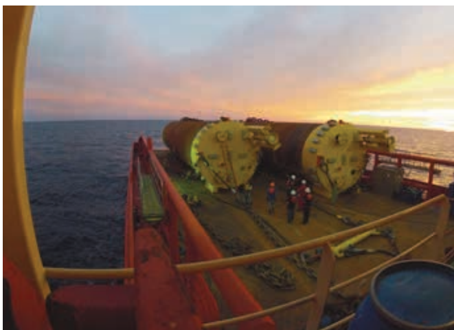
Figure 3. Employees review rigging and procedures one last time before over-boarding a suction pile for installation in the Delta House mooring system.
