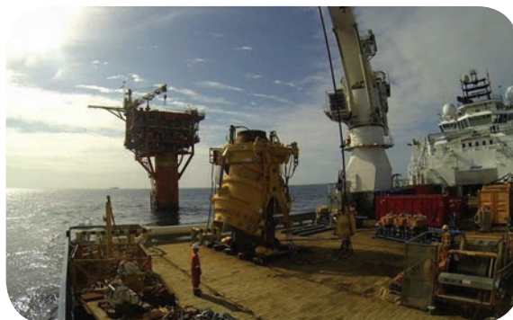
The clamp on deck, with the Varg A monotower in the background. Photos from IK.
